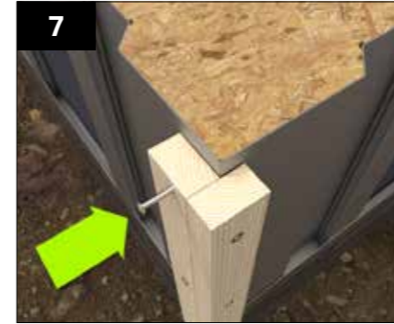
At corners battens should be fixed as shown. This ensures that claddings at the corners are well reinforced.
