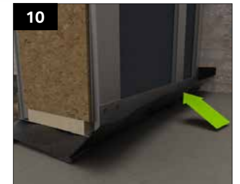
Internally fold up the excess DPC and temporarily fix in place, this can be done with tape or other method.
